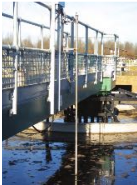
VIPER TRANSDUCER ON CONDUIT WITH ROTATING BRIDGE
