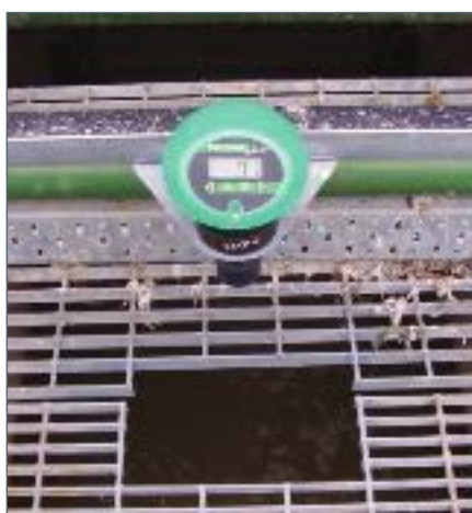
IMP CONTROLLING GATE HEIGHT
