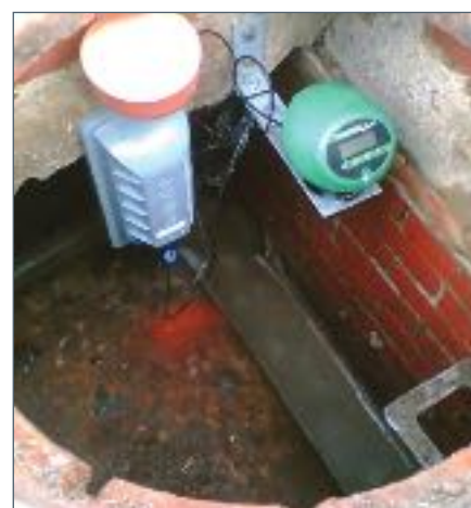
IMP MONITORING IN A CSO CHAMBER
