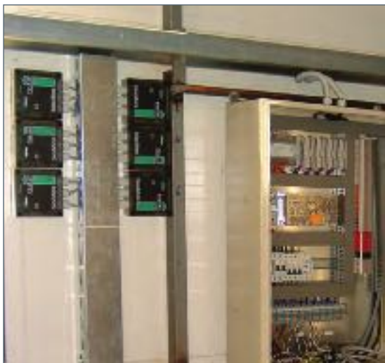
MINERAL OIL TANK LEVEL
