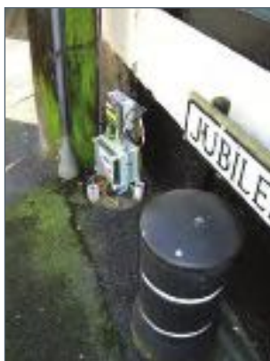
LEVEL CSO MOUNTED ON BATTERY PACK INSIDE A BOLLARD
