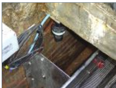
dB3 WITH DRIP SHIELD MOUNTED IN CSO CHAMBER
